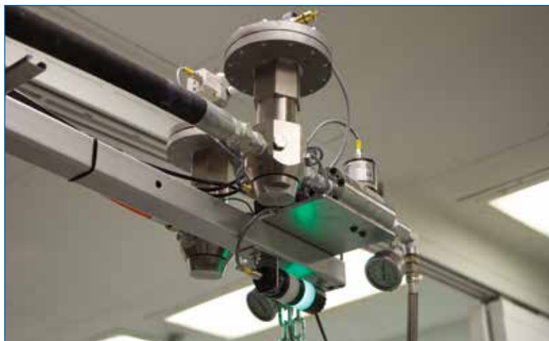
The system's green light tells you that materials are being dispensed on-ratio.
